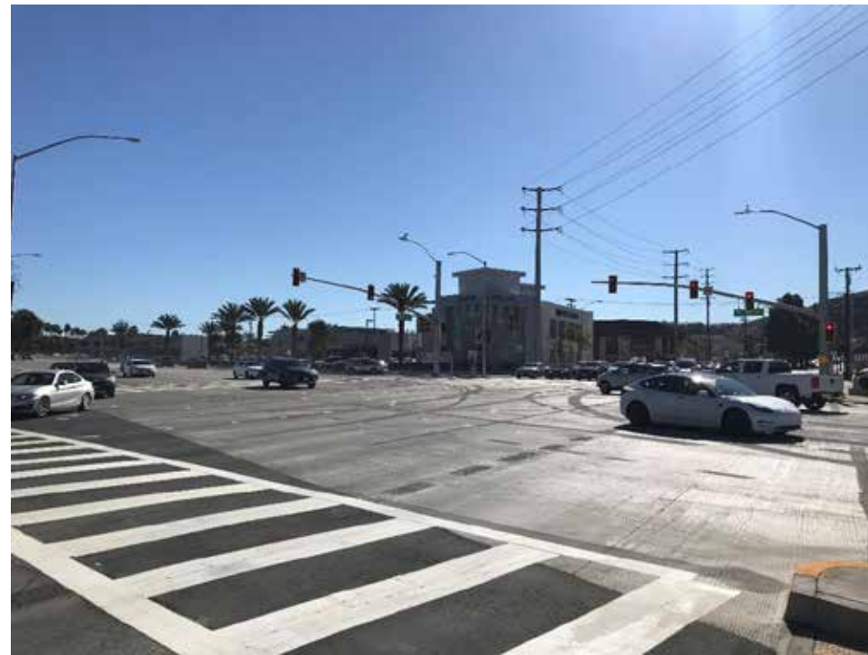
Completed concrete pavement and widened intersection looking southeast across Pacific Coast Highway.
