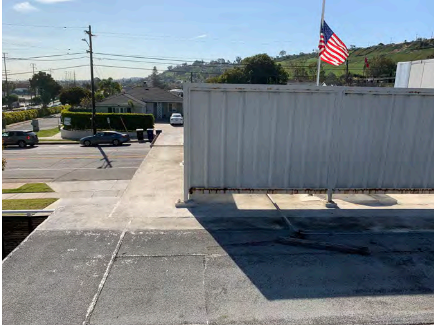
Non-lead gray gate paint.
