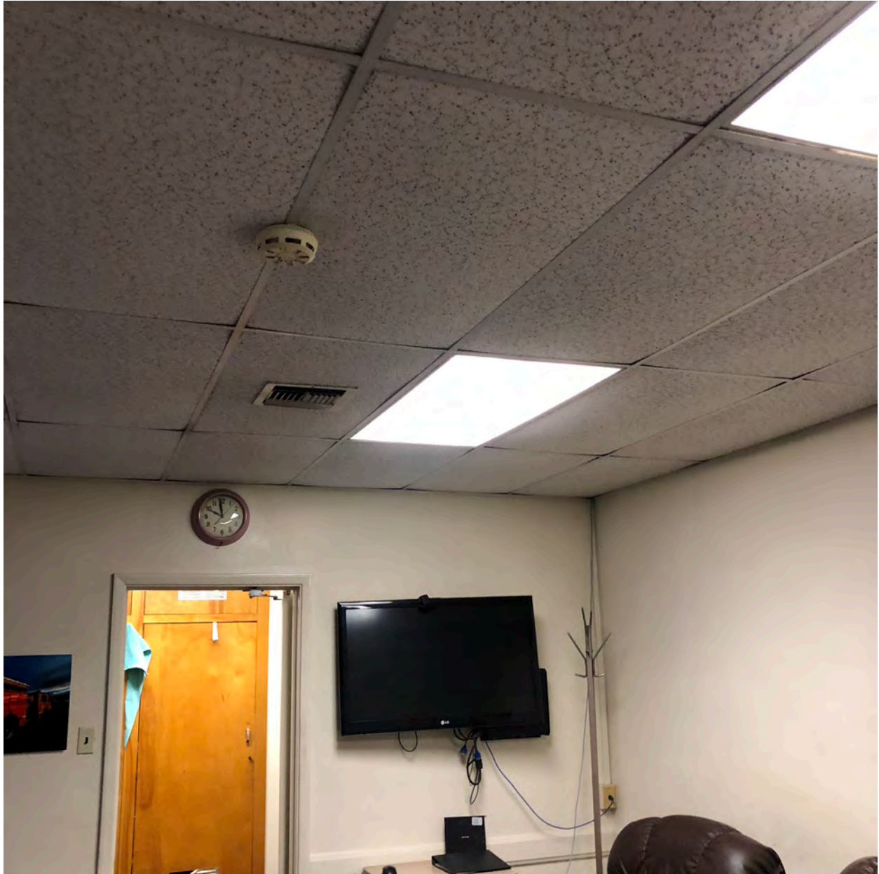
White wall paint in the dorm and rec. room is lead-based.
