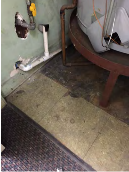
Brown 12" tile and mastic – 5% asbestos
