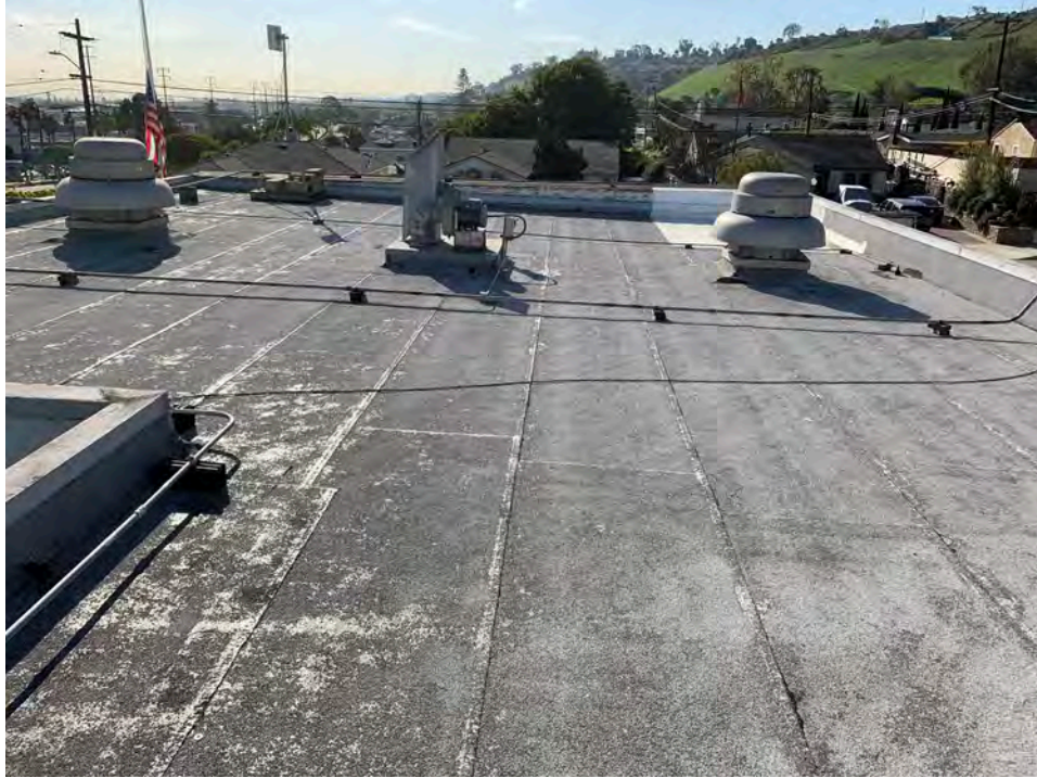
ACM pedestal mastic – center roof.
