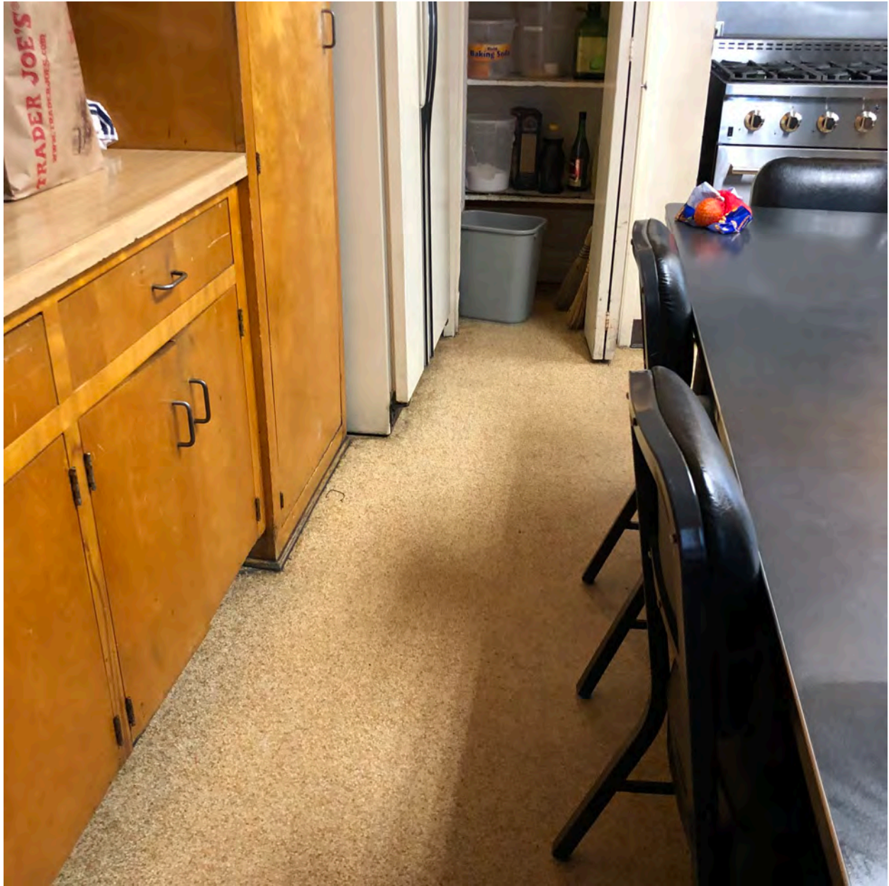
Asbestos containing floor mastic and sheet flooring in the kitchen.
