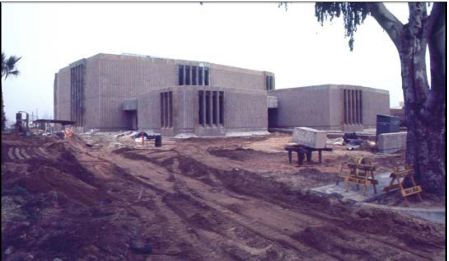
The construction of the Civic Center Library in the 1970s was a major addition to the complex of City facilities and offices along Torrance Boulevard at Madrona Avenue.
