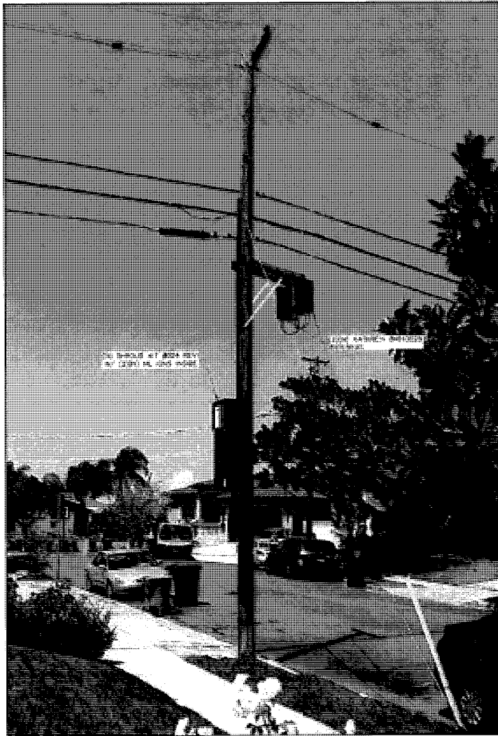
Figure 1: Proposed node on existing utility pole.
