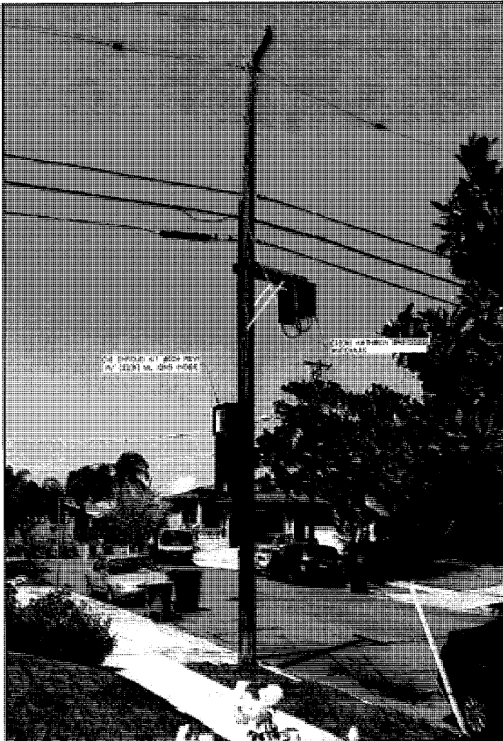
Figure 1: Proposed node on existing utility pole. (Source: Applicant's Photo Simulation submitted through the January 23, 2018 submission).
